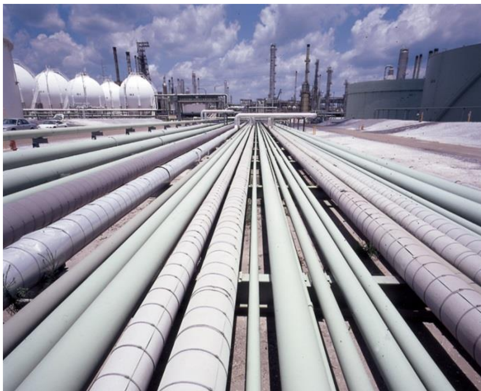
Figure 16. Above ground oil pipelines.
